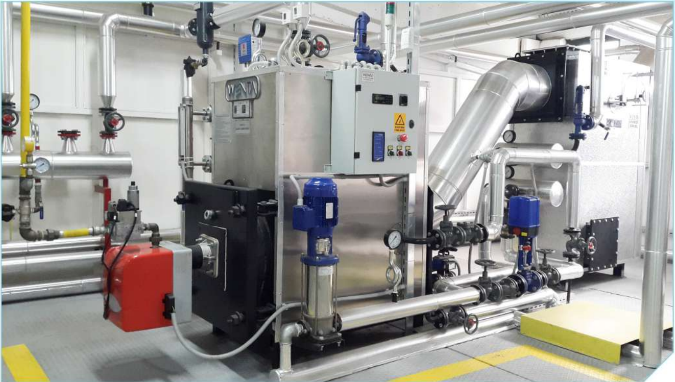
Örnek Ekonomizer uygulaması WENTA Fabrikası/ANKARA 2017. An example of Economizer application in WENTA Factory/Ankara 2017.
